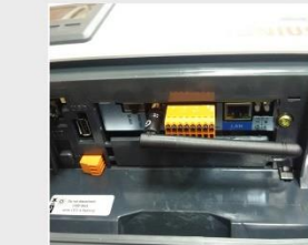
Figure (2). An overview of Datamanager installed in a single phase inverter(WiFi antenna, LAN port, LED indicator lights and Master / Slave switch or Datamanager on / off are visible)
